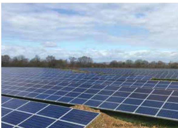
Photo Courtesy by ENGIE Fabricom
