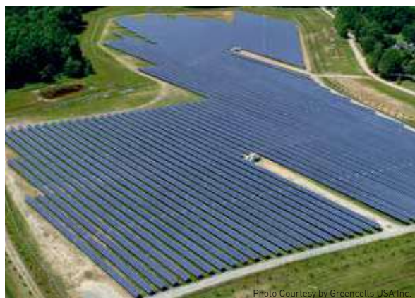
Photo Courtesy by Greencells USA Inc.
